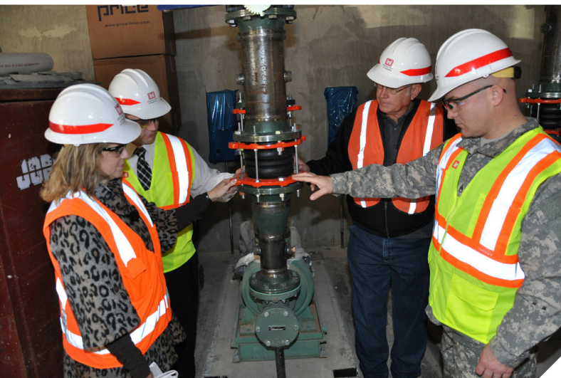
Louisville Ground Source Heat Pump. CREDIT: U.S. Army Corps of Engineers
