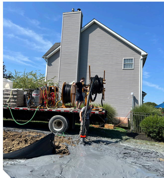
Members of United Association of Plumbers and Steamfitters Local 7 install a TEN at Saratoga County Airport. CREDIT: United Association of Plumbers and Steamfitters Local 7
