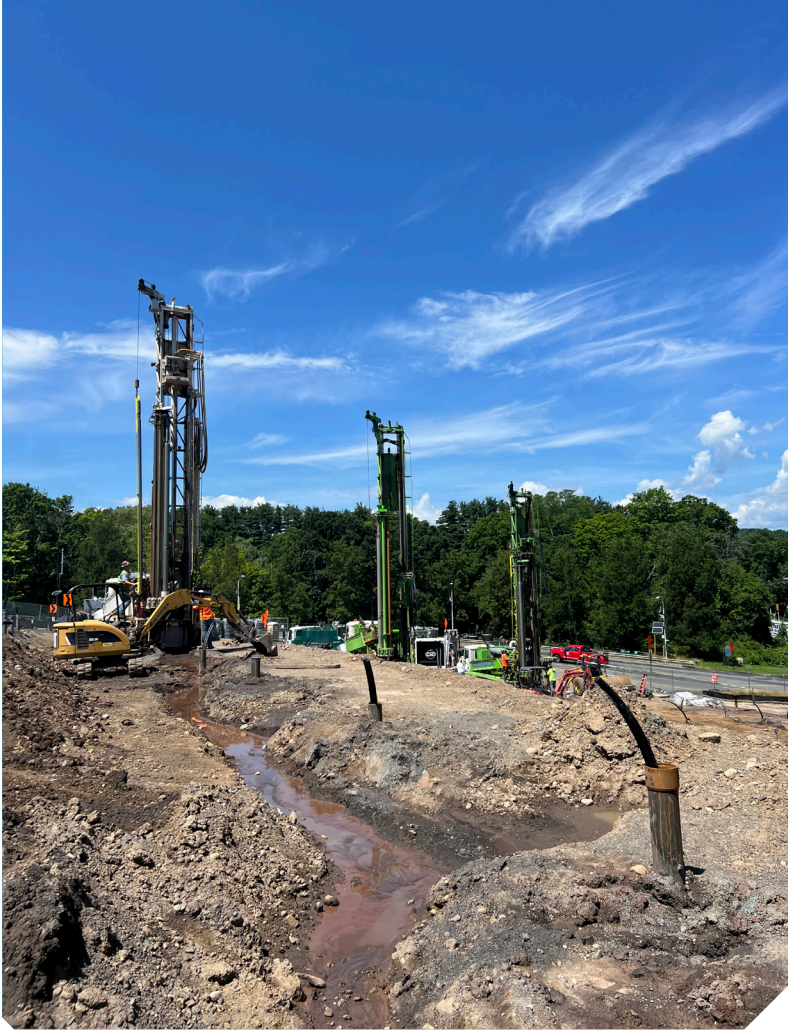
Installation of a TEN at Saratoga County Airport. CREDIT: United Association of Plumbers and Steamfitters Local 7
